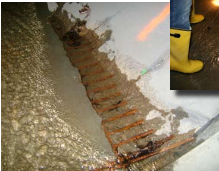
You can see the cracking and exposed re-bar on the original RCP.
