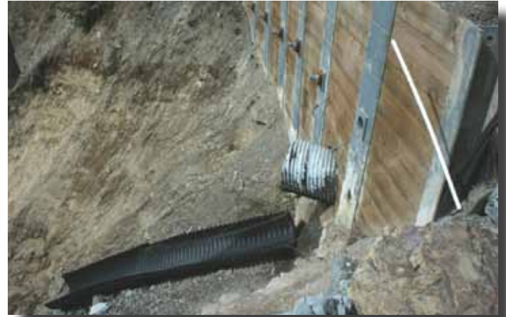
Figure 1: The 36-inch CMP with a half-pipe included as a temporary fix to the failing culvert.
