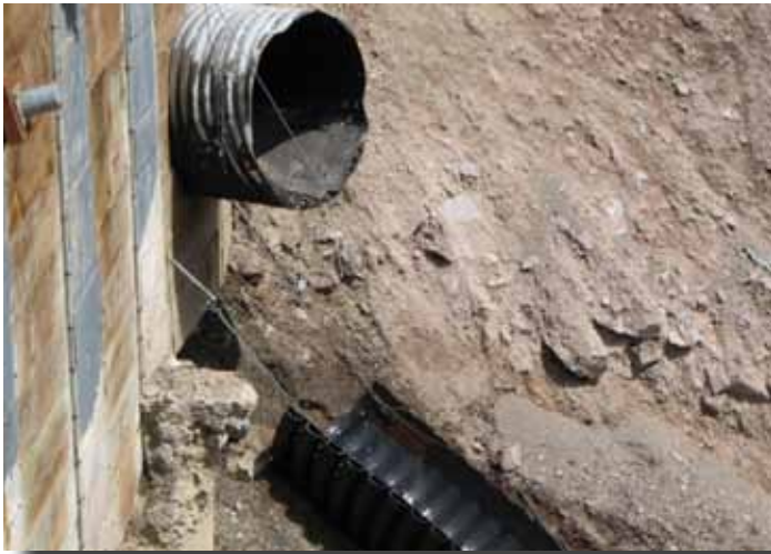
Figure 3: Outfall at the soldier pile wall showing the exposed lagging
