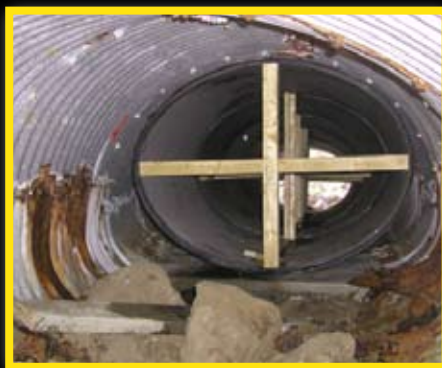
Above: Snap-Tite pipe coming through a deteriorating culvert during installation (struts will be removed once completed).
